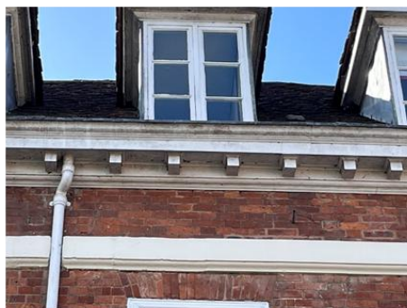
Saw tooth dentilling (top left), Hit and miss header dentilling (top right), High quality eaves treatment (bottom)
