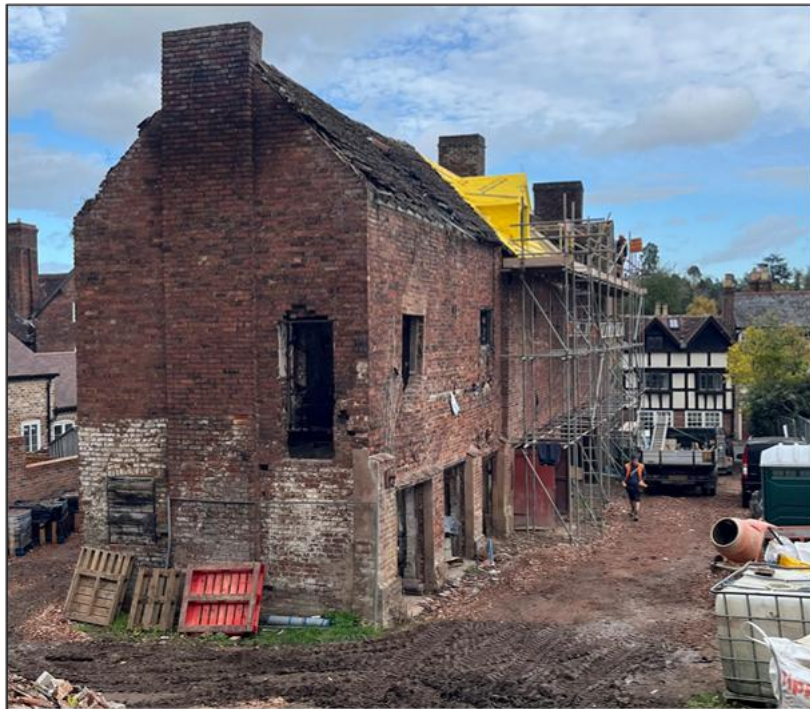
Old Workhouse, High Street. A programme of restoration has been agreed.
