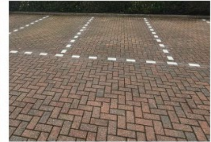
Parking bay demarcation with white lines.
